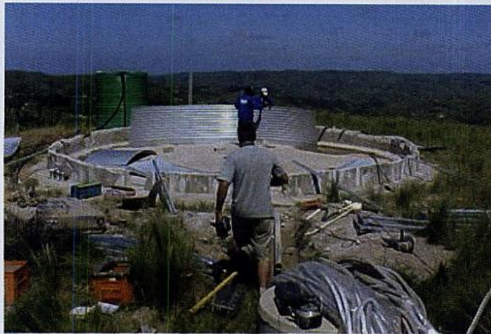
Installation of Galaxy Reservoir inside the 'old reservoir' footprint – panels had to be carried up the hill to final location
