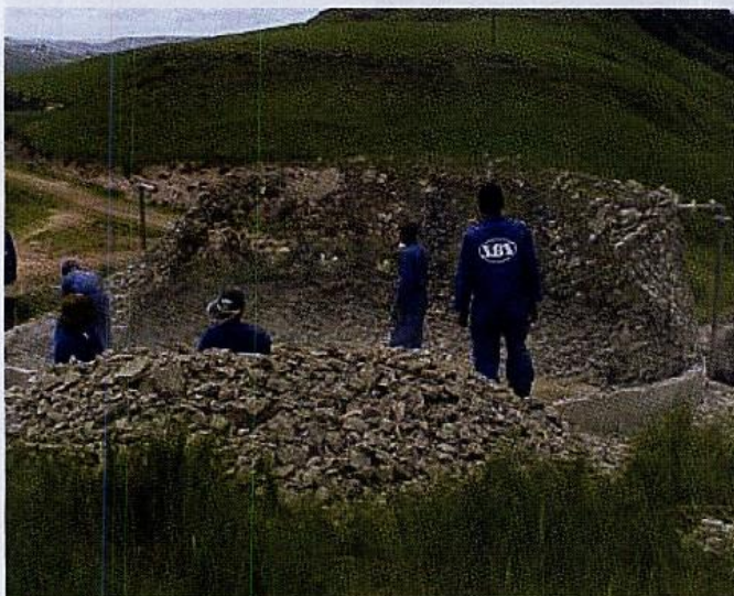
Above pictures show demolishing of reinforced ferrocement reservoirs, walls demolished to floor level, leaving concrete base only
