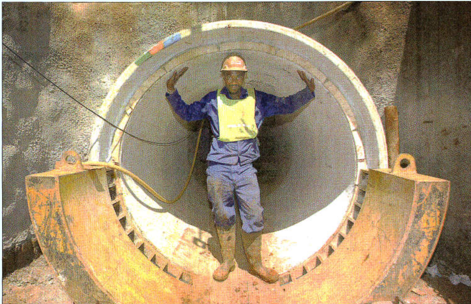
A worker demonstrates the size of the award-winning concrete sleeve constructed on Town Hill to house a new water pipeline for Umgeni Water.
