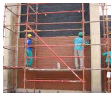
Figure 3: Brickwork inner and outer face on panels at northern end pump station
