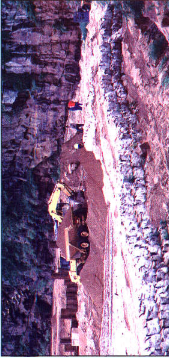
Contract workers are seen re-building the Umvoti River bank which collapsed after the flash floods on Thursday and Friday
