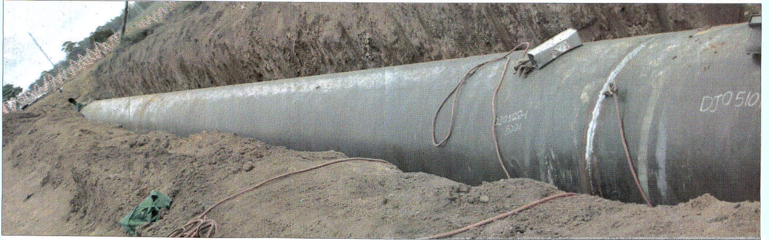
MAJOR PROJECT: Pipes being laid in the Cato Ridge area on private property. Here, important grasslands were identified and the team tried to reduce the environmental impact.
