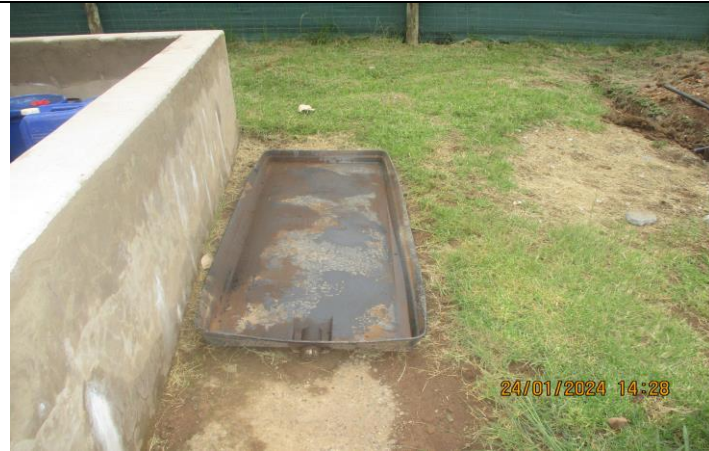
Figure 2: Drip tray needs to be replaced
